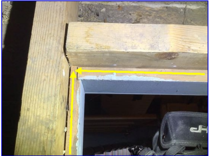
Suggest installation of weatherstripping annually at attic hatch to reduce build up of warm moist air which often causes moisture issues.
