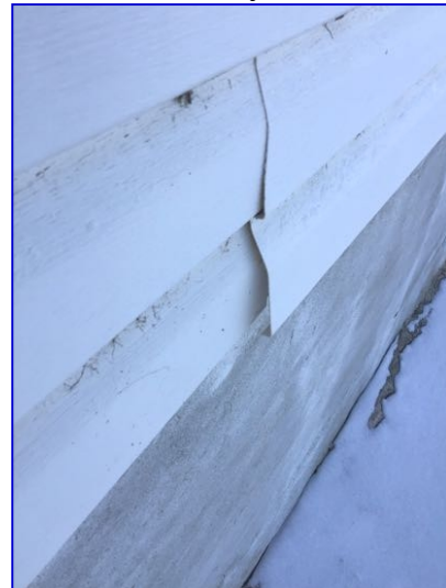
Loose siding noted. Suggest securing to prevent water entry and wind damage.
