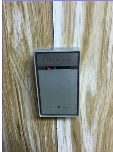
Thermostat secure on wall and functional on day of inspection. Located at Main Level hallway
