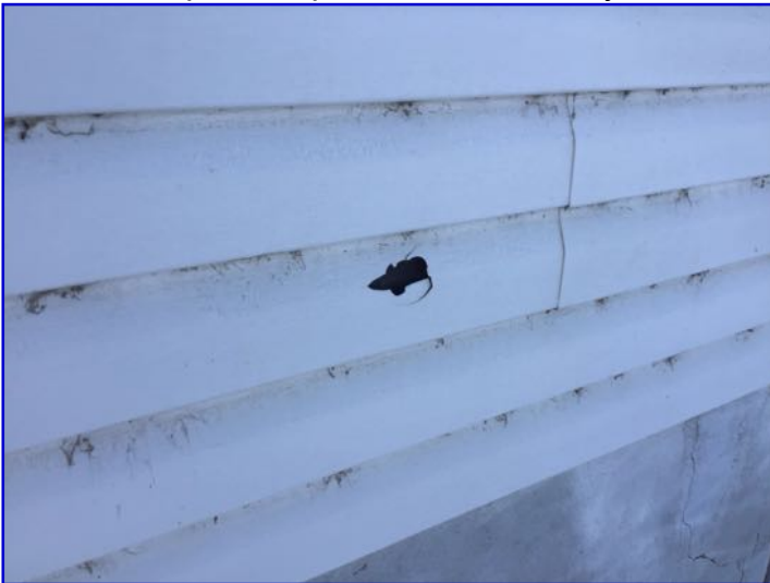
Areas of damage noted to wall cladding.
