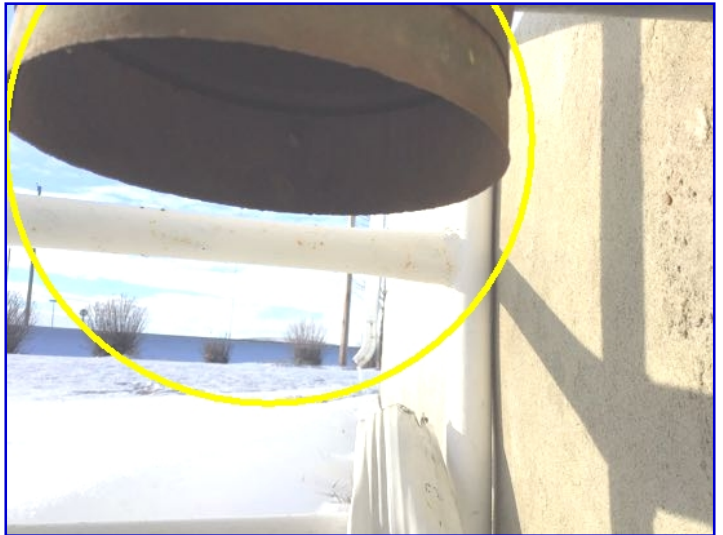
Missing cap at exhaust venting. Replace to prevent down drafting
