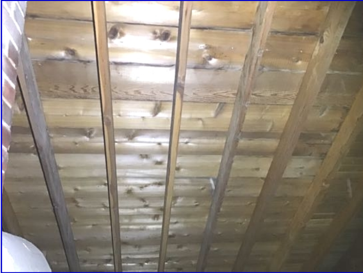
The sheathing was visually inspected and appeared dry on the day of the inspection. (we can only comment on what is visible and accessible areas from the attic hatch at the ladders edge)
