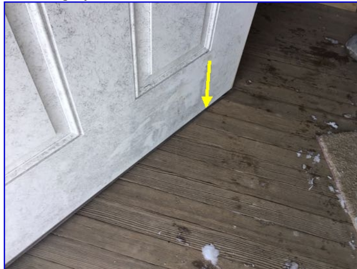
Mudroom door scrapes on floor. Recommend adjustments as required.
