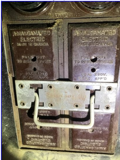
Amalgamated fuse blocks noted. Replace with more current breakers for safety.
