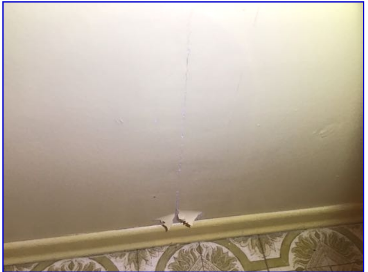
Areas of cracking / peeling noted at Bathroom walls.
