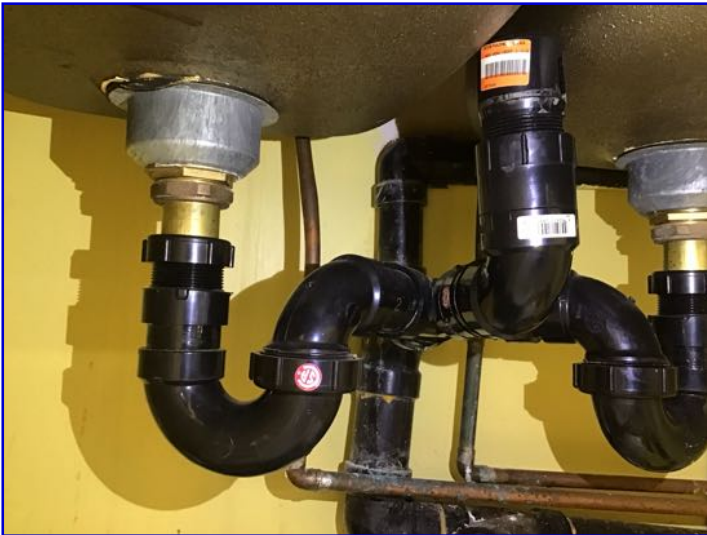
No water supply shut offs noted. Recommend review of waste line installation.
