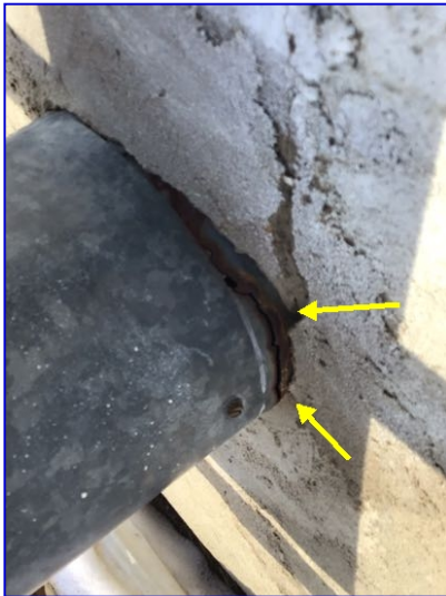
Rust / holes noted in venting. Repair for safety.
