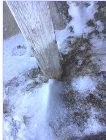
Post deterioration noted at porch / Mudroom framing.
