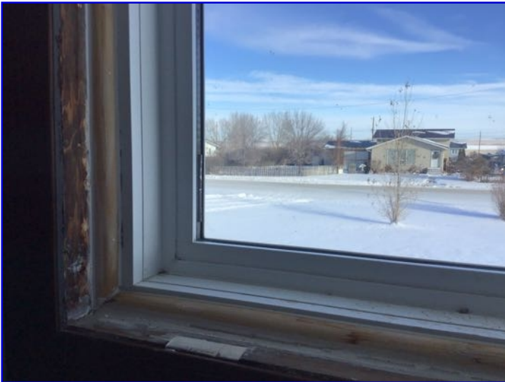
Water staining observed at sills. Recommend monitoring and maintaining to prevent possible water damage
