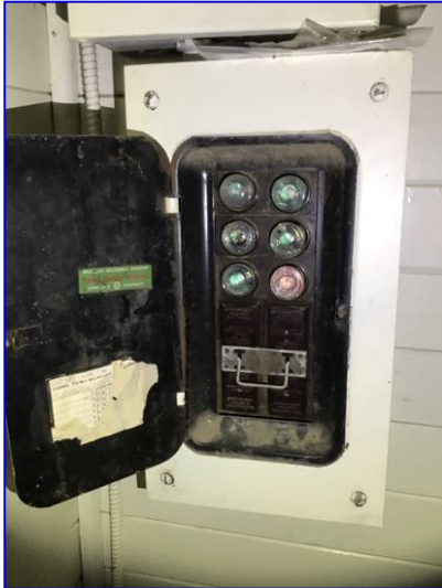
Outdated panel noted. Recommend further review for replacement by qualified electrician.
