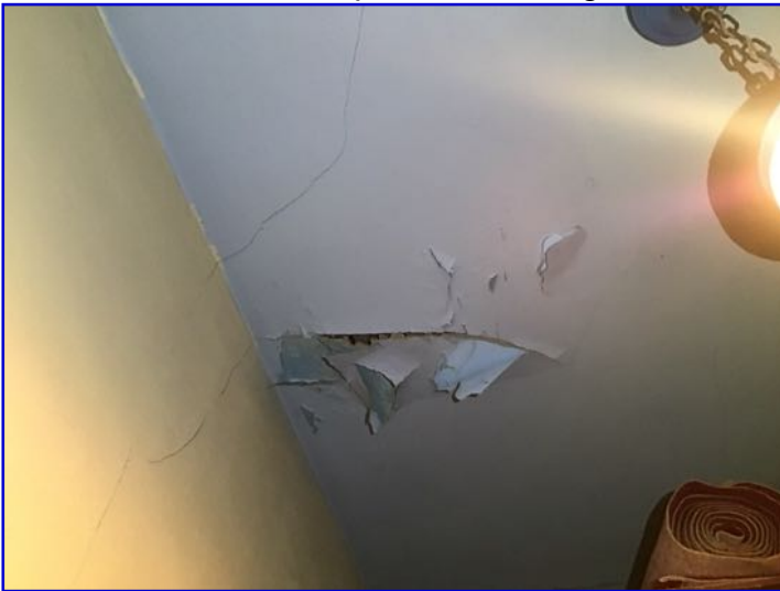
Blown out ceiling plaster noted. Recommend repairs
