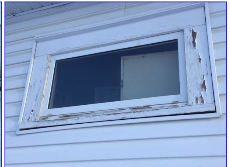
Peeling paint noted. Maintain all exterior wood
