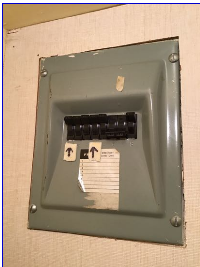
Sub Panel located in the bathroom.
