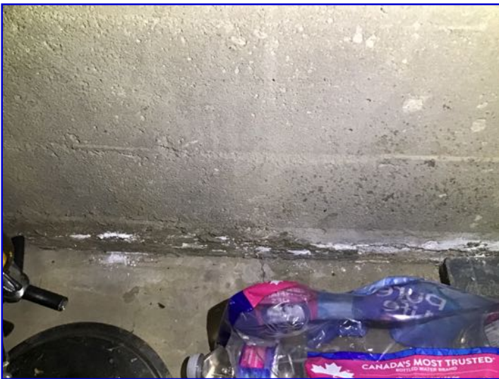
Efflorescence observed at walls / slab. This is a white mineral deposit left behind from water infiltration.
