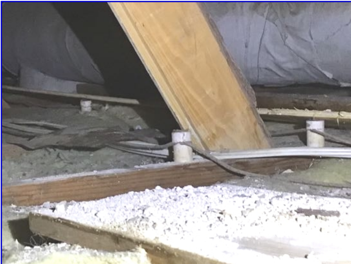
Further review by qualified electrician recommended for safety.
