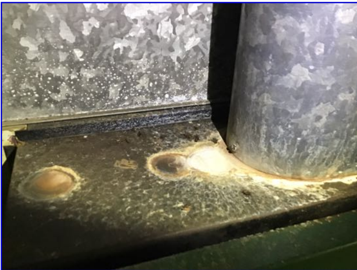
Recommend further review of furnace.
