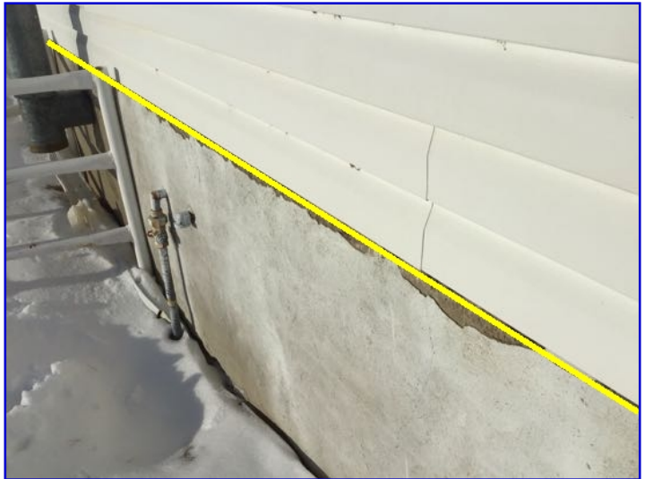
Recommend installing flashing to prevent water entry.
