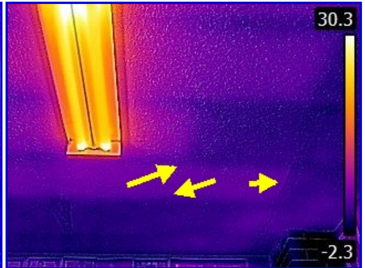
Cold areas noted at basement ceiling
