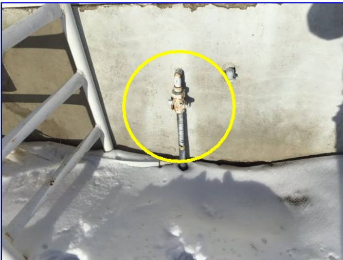
Gas shut off valve at rear of building.
