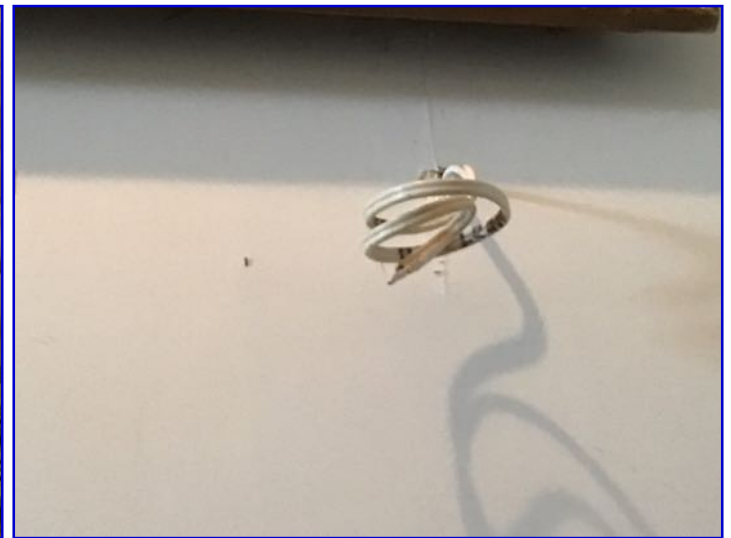
Exposed electrical wiring observed. Client should consult with a licensed electrician prior to closing for repairs/replacement as needed to ensure safety.
