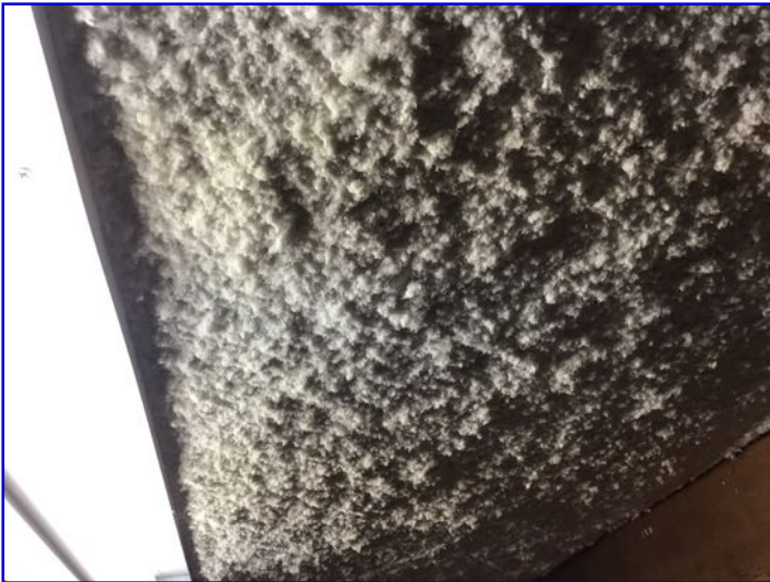
Exposed styrofoam / foam spray observed. This material should be covered with drywall or other fire rated material for safety.
