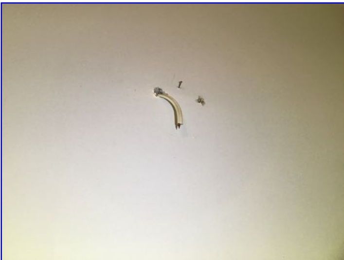
Repair exposed wiring for safety.
