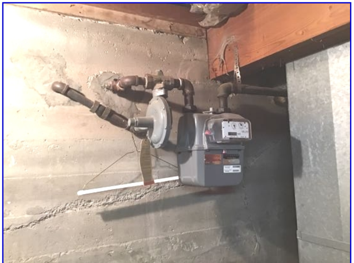
Gas meter is located in the furnace room - this is the main gas shut off to the home
