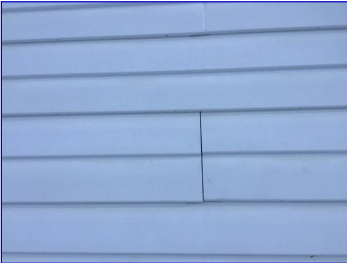
Gaps noted in vinyl siding. Recommend adjusting to prevent possible water entry.
