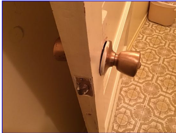
Bathroom handsets loose and require tightening.
