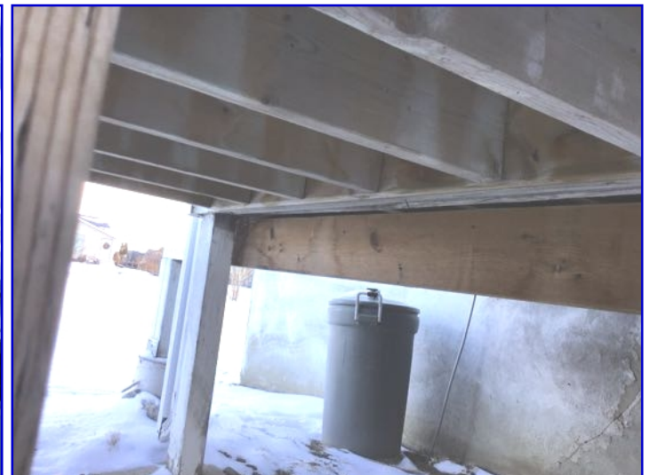
Recommend further review of porch area framing.
