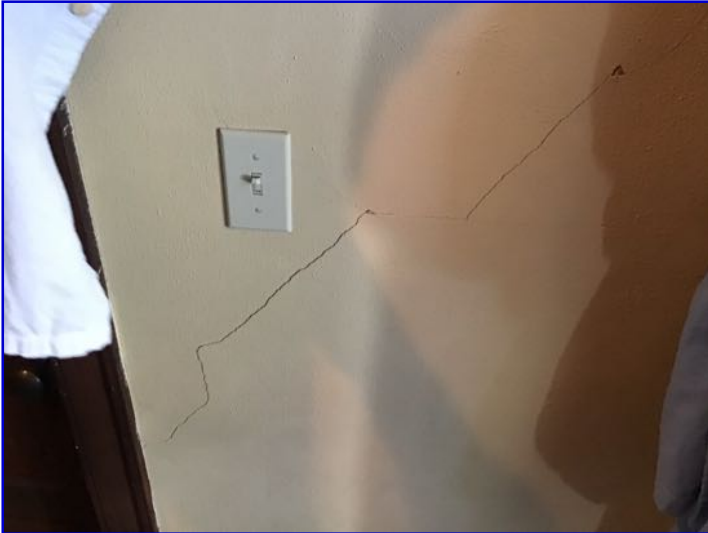
Several areas of plaster cracking noted
