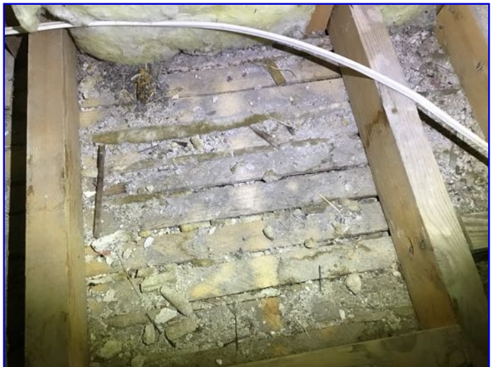
Missing insulation noted in several areas of attic. Add as required
