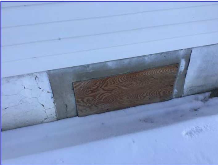
Several abandoned windows boxed in noted.
