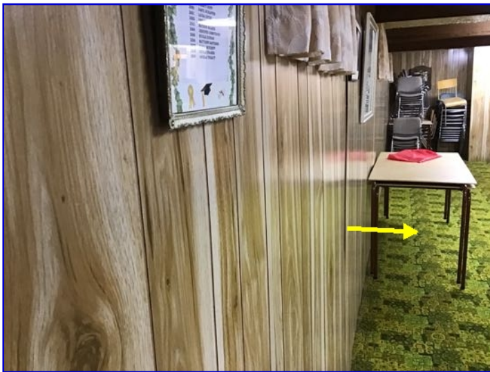
Bowing / loose wall panelling noted in areas.
