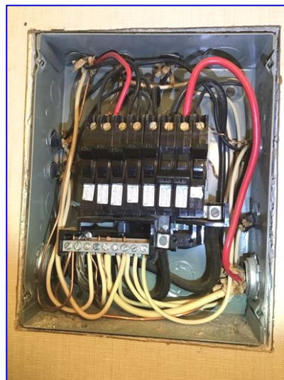
No major causes for concern noted at the sub panel.
