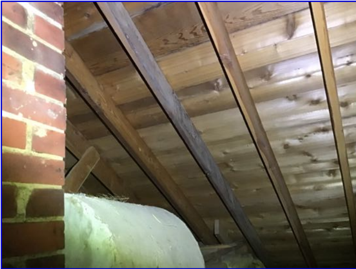
Attic should be reviewed at least twice per year to ensure ventilation openings are clear and to ensure development of organic growth is kept in check
