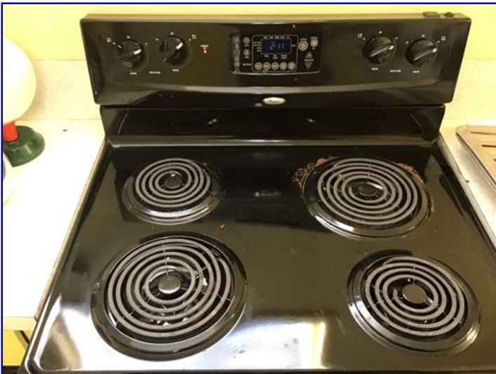
Stove elements slow to heat but working at time of testing.
