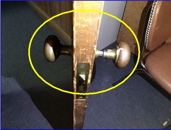
Door hand sets require attention.
