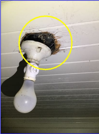
Loose fixtures noted. Secure for safety.
