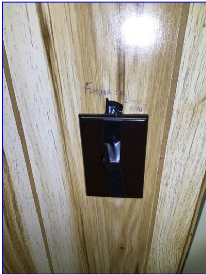
Furnace electric disconnect switch
