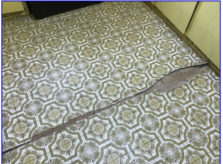
Kitchen floors in fair to poor condition - Visual damage noted to floor surface
