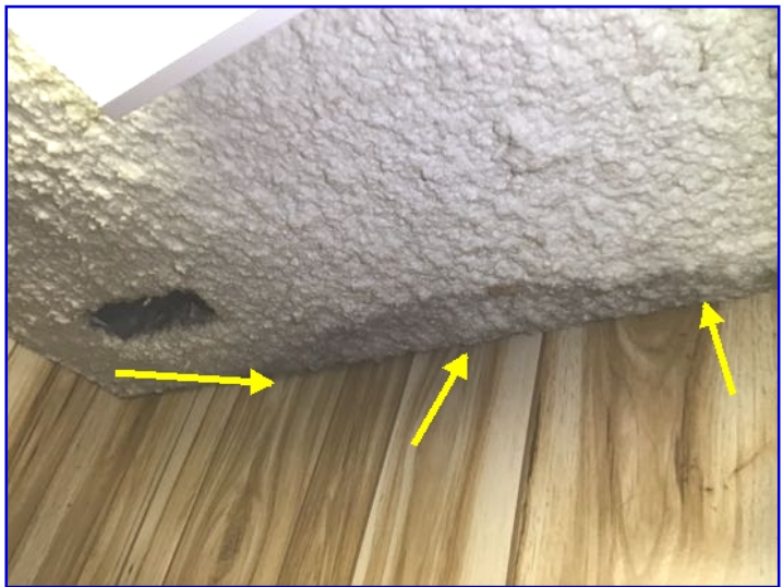
Areas of staining noted.
