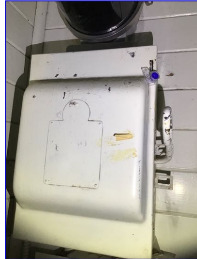
Main electrical disconnect / shut off
