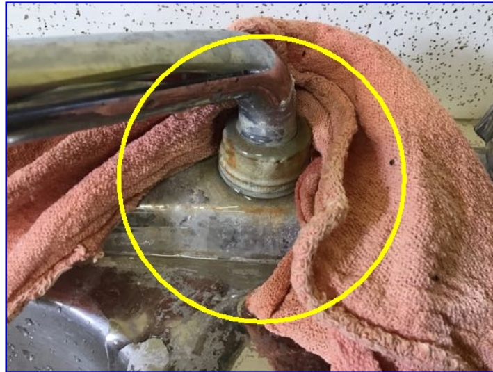
Faucet is leaking. Repair/replace as required. Water damage will occur to counter top if left leaking.
