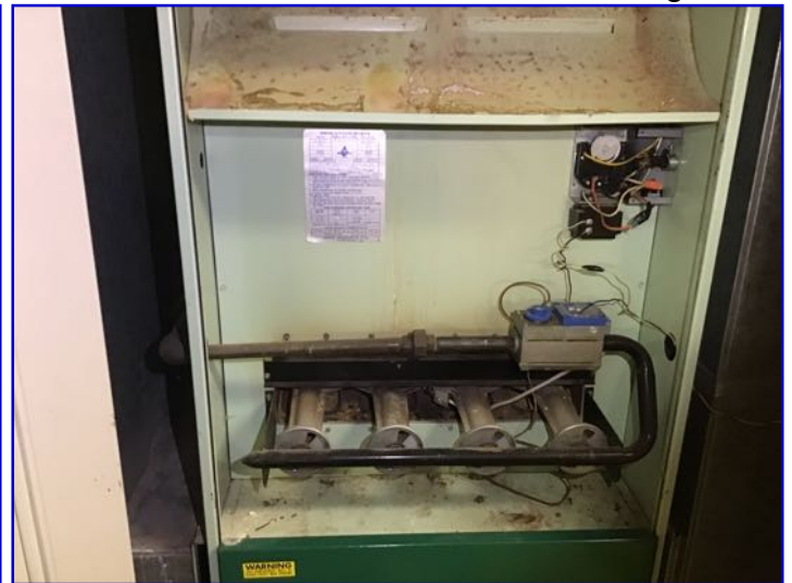
No record of recent service observed. Recommend cleaning and service by a qualified HVAC contractor on possession, and annually thereafter for efficient operation of system.
