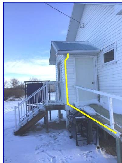
Ensure water is directed away from structure
