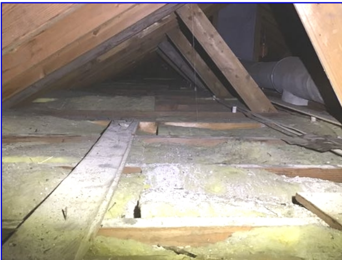
Suggest adding additional insulation in the attic to reduce heat loss.
