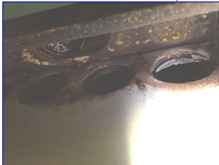
Recommend further review of heat exchanger by qualified furnace technician.
