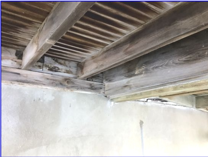
Recommend review of Mud Room framing to confirm structural integrity.
