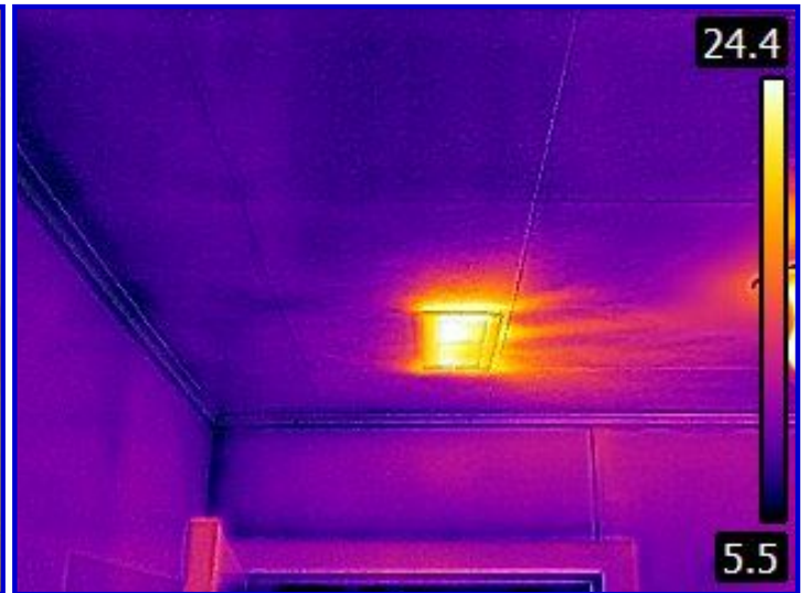
Main Washroom ceiling dry on Thermal scan
