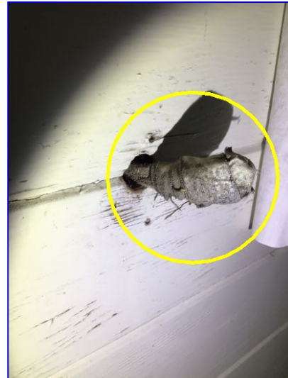
Proper termination of wiring is recommended for safety.
