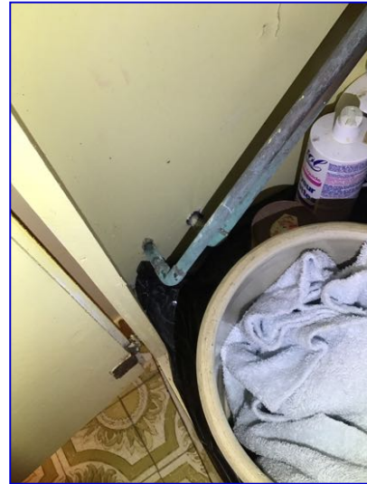
Corrosion observed at copper supply lines.
