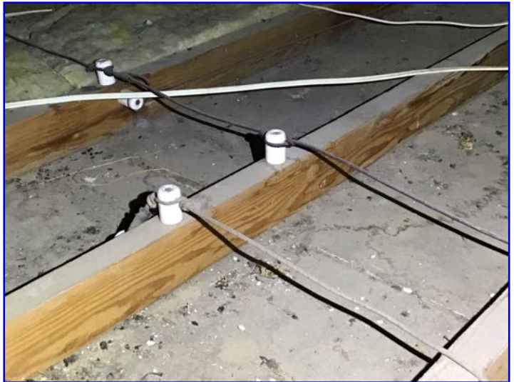
Recommend full review of electrical system by qualified electrical contractor for quotes on upgrades/repair to ensure safe and adequate service.
