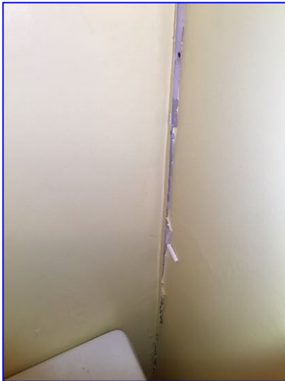
Cracking noted at Bathroom walls.
