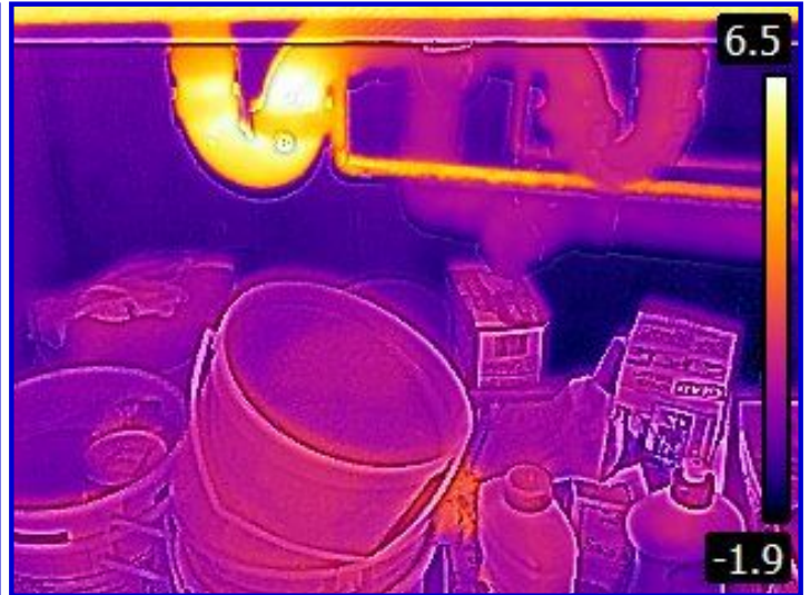
No leaking noted at Kitchen sink cabinet on Thermal image
