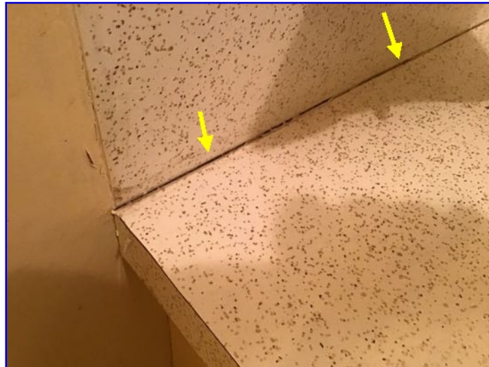
Faucets were run for a period of time. No leaks observed unless otherwise noted. Aerators Recommend regular caulking to prevent water entry behind the waterproof surface.
