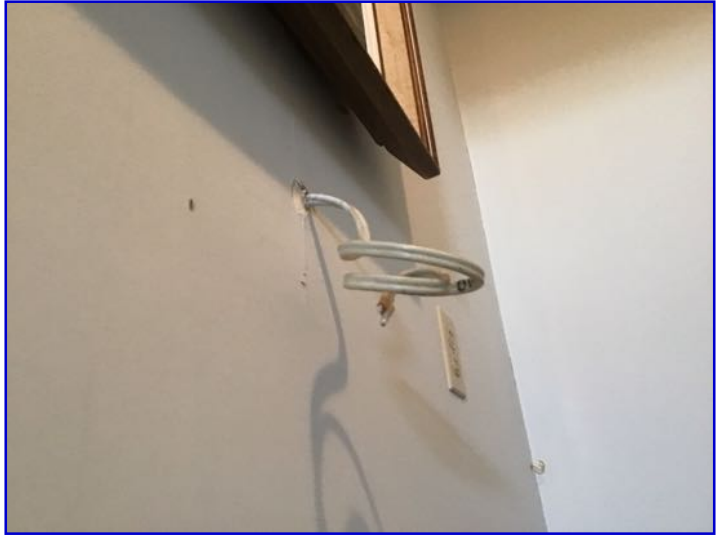
Exposed electrical wiring observed in areas. This is a safety concern as it is subject to "Physical Damage". Exposed electrical wires should be encased in protective cable cover to ensure safety from mechanical damage. Client should consult with a licensed electrician prior to closing for repairs/replacement as needed to ensure safety.
