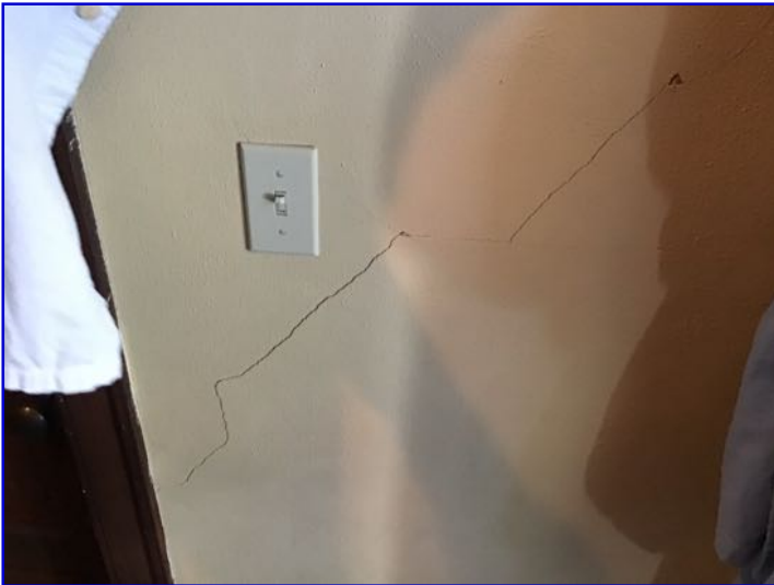
Several areas of plaster cracking noted
