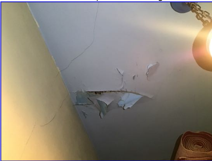
Blown out ceiling plaster noted. Recommend repairs
