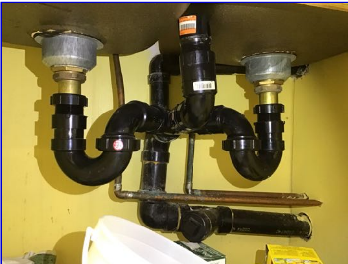
No leaks at traps or drains observed. Water was run for some time to fully test for problems. In some cases plumbing venting is not visible as located inside the wall. Concealed areas excluded as part of the inspection.
