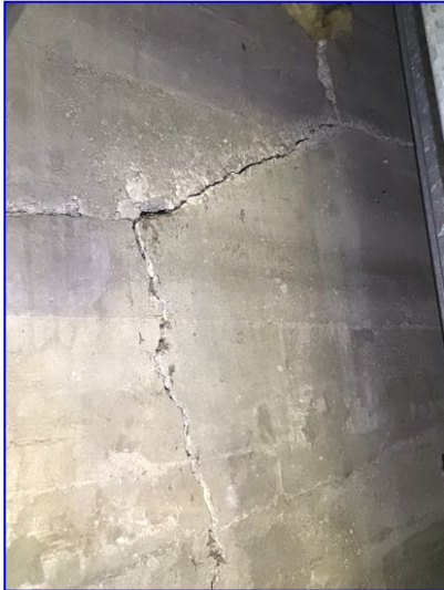
Cracking noted in several areas of interior foundation walls. Repair to prevent water entry.
