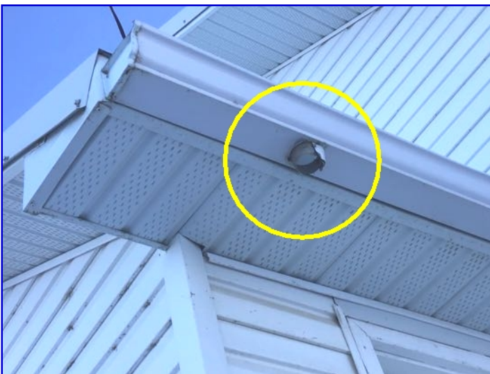
Missing downspouts observed. Suggest downspouts be installed to ensure proper drainage away from the foundation.
