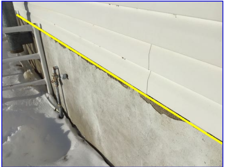
Recommend installing flashing to prevent water entry.
