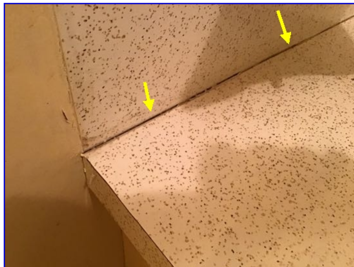
Faucets were run for a period of time. No leaks observed unless otherwise noted. Aerators Recommend regular caulking to prevent water entry behind the waterproof surface.
