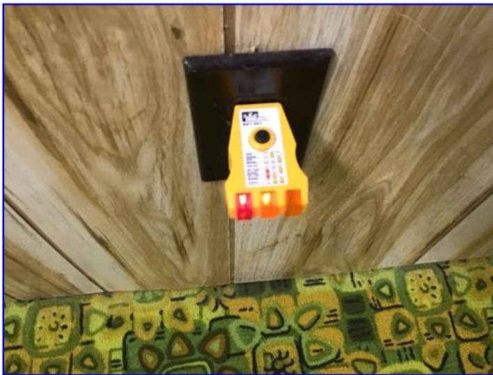
Reverse polarity observed at receptacles in basement. Recommend addressing by a qualified electrician
