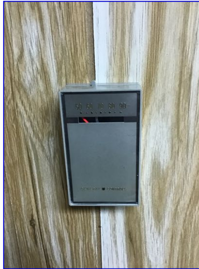
Thermostat secure on wall and functional on day of inspection. Located at Main Level hallway
