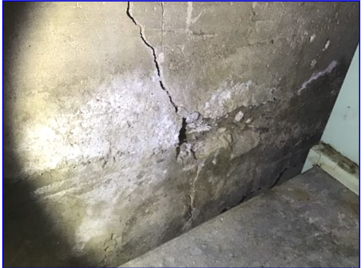
Deterioration noted at areas of the concrete foundation walls. This is often seen with the older homes. Concrete foundations have an approximate life of a hundred years. Due to the condition of the foundation, we recommend full review by a qualified basement contractor prior to close.
