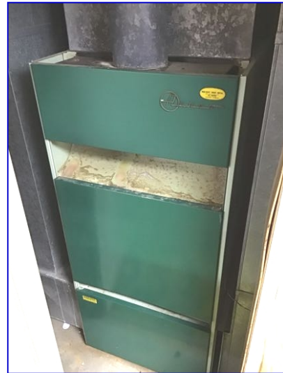
ATCO gas provides a free safety inspection of gas burning appliances. This is strongly recommended for this furnace due to it's condition / age.
