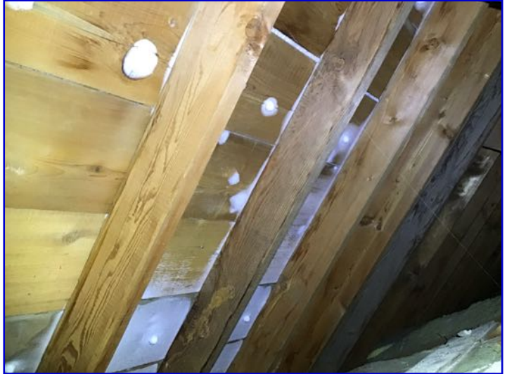
Frost / ice build up noted at sheathing and framing - Common causes are heat loss into attic area and or poor ventilation. This can cause moisture to drip onto ceiling below resulting in staining when temperatures warm up and melts frost / ice. This phenomenon is often referred to as attic rain.
