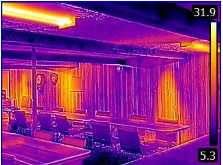
Basement right - Thermal Image
