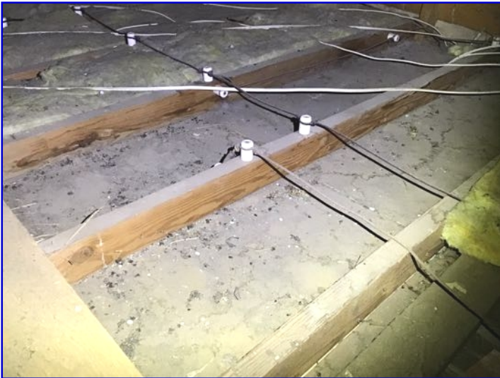
Knob and tube wiring was observed in this home. This type of wiring was standard at the time of construction. Recommend further review by qualified electrician for safety.
