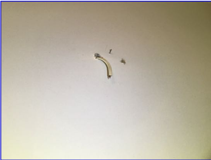
Repair exposed wiring for safety.
