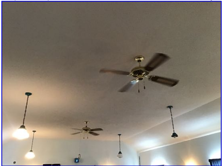
Ceiling fans in hall noisy when operating.
