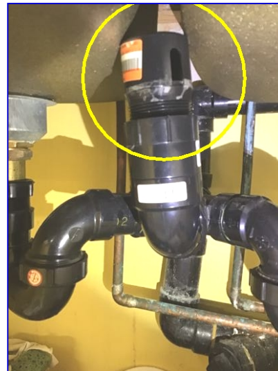
Air Admittance Valve vent observed at waste line. These devices are installed in islands when venting is difficult. Installation of AAV should be installed above flood rim of sink.
