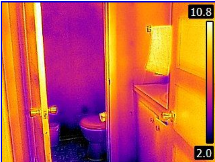
Main Washroom - Thermal Image
