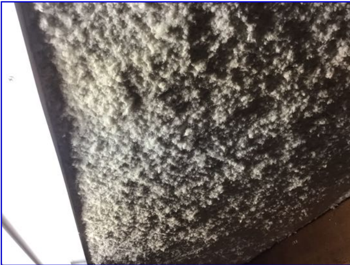
Exposed styrofoam / foam spray observed. This material should be covered with drywall or other fire rated material for safety.
