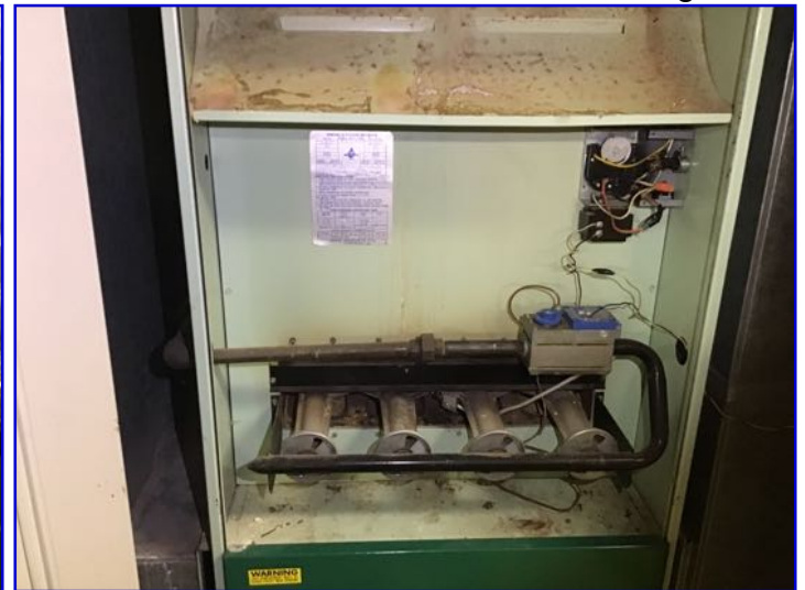
No record of recent service observed. Recommend cleaning and service by a qualified HVAC contractor on possession, and annually thereafter for efficient operation of system.
