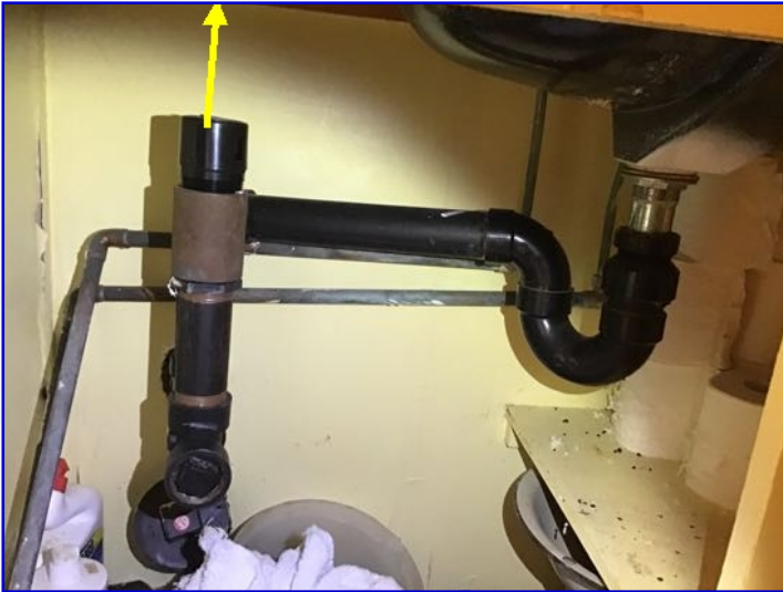
Air Admittance Valve vent observed at waste line. Installation of AAV should be installed above flood rim of sink.
