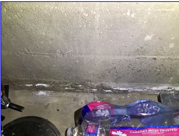
Efflorescence observed at walls / slab. This is a white mineral deposit left behind from water infiltration.
